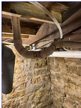
Shower drain has an up hill flow and may cause drainage issues.
