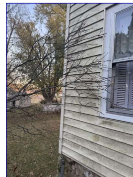
Tree branches rubbing on siding.
