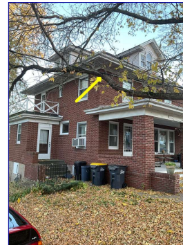
Recommend a licensed electrician/utility company trim the branches away from the roof electric supply lines to the house. This is a safety concern.
