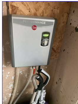
The Water Heater Area located in laundry room.
