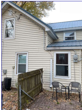
The electrical service drop
