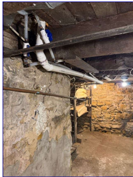
The visible drain/waste piping
